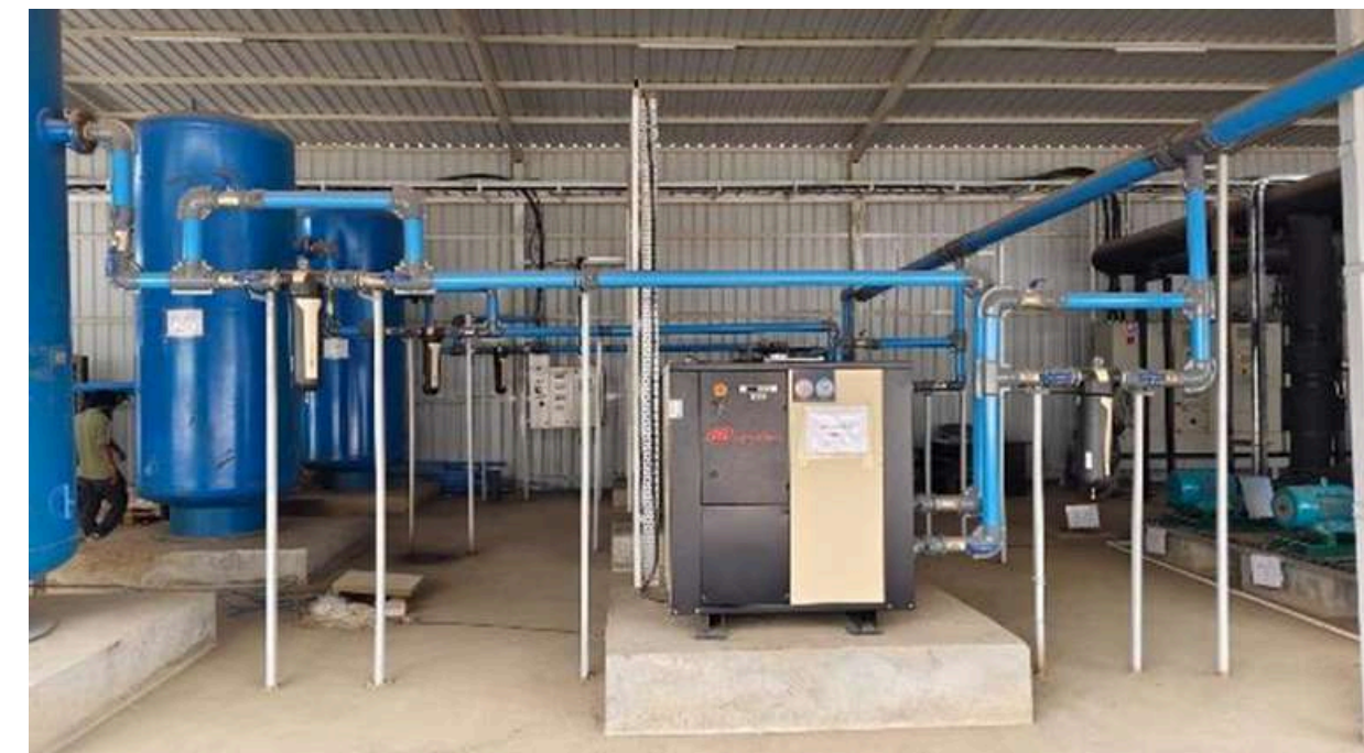
Compressor with Compressed Air Piping
