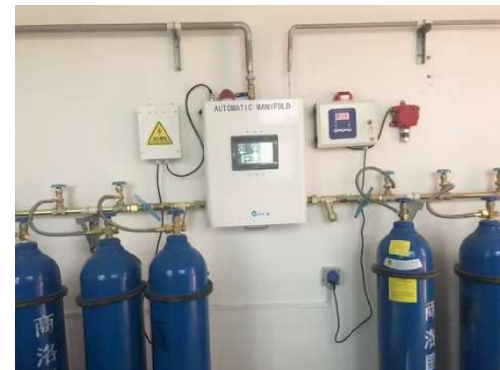
Oxygen Cylinder Gas Bank
