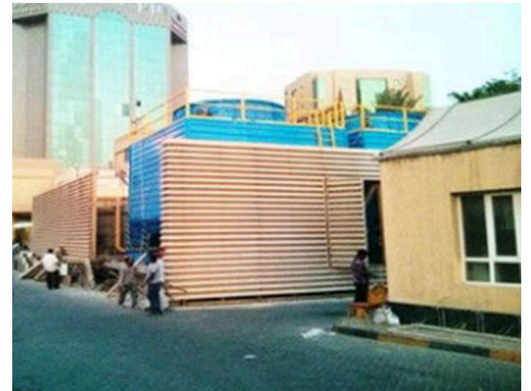
4 Cell Cooling Towers
